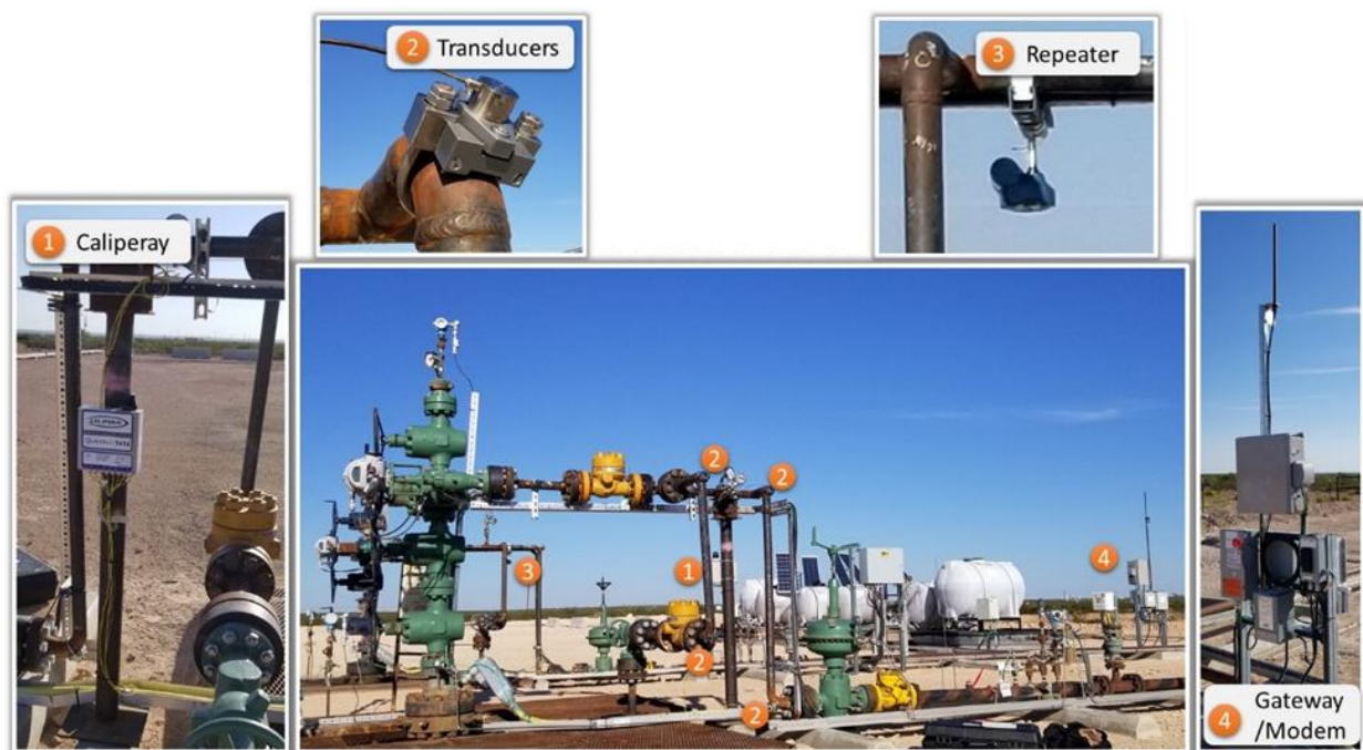
Figure 1: The system configuration and sensor install locations.
