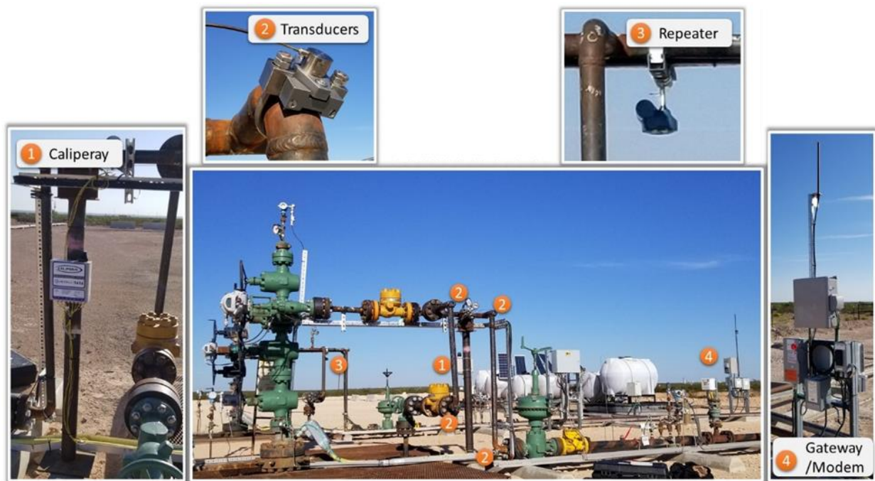
Figure 1: The system configuration and sensor install locations.
